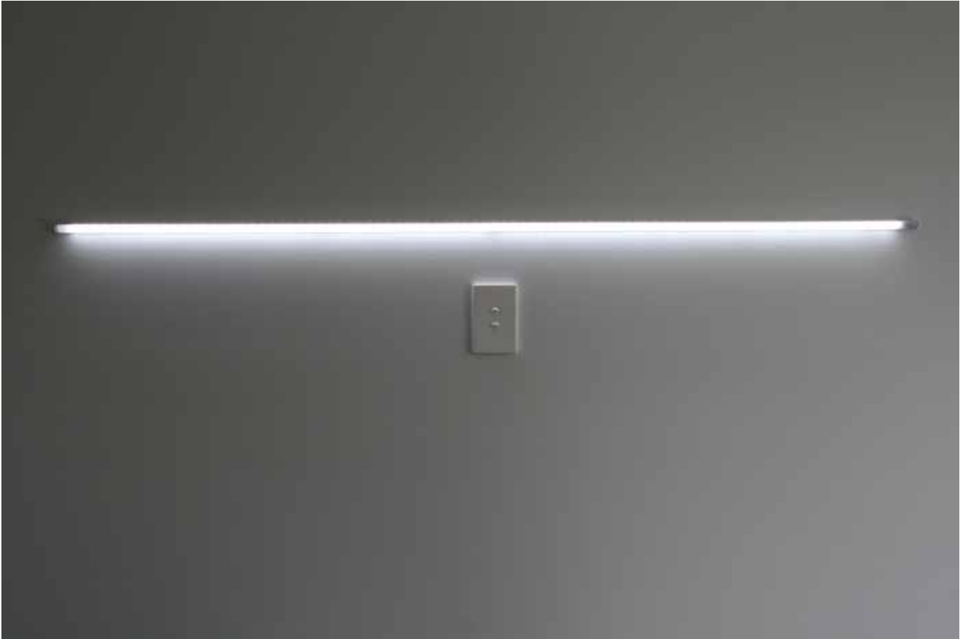
Strip Light in corner channel, used as a wall light above a bed
