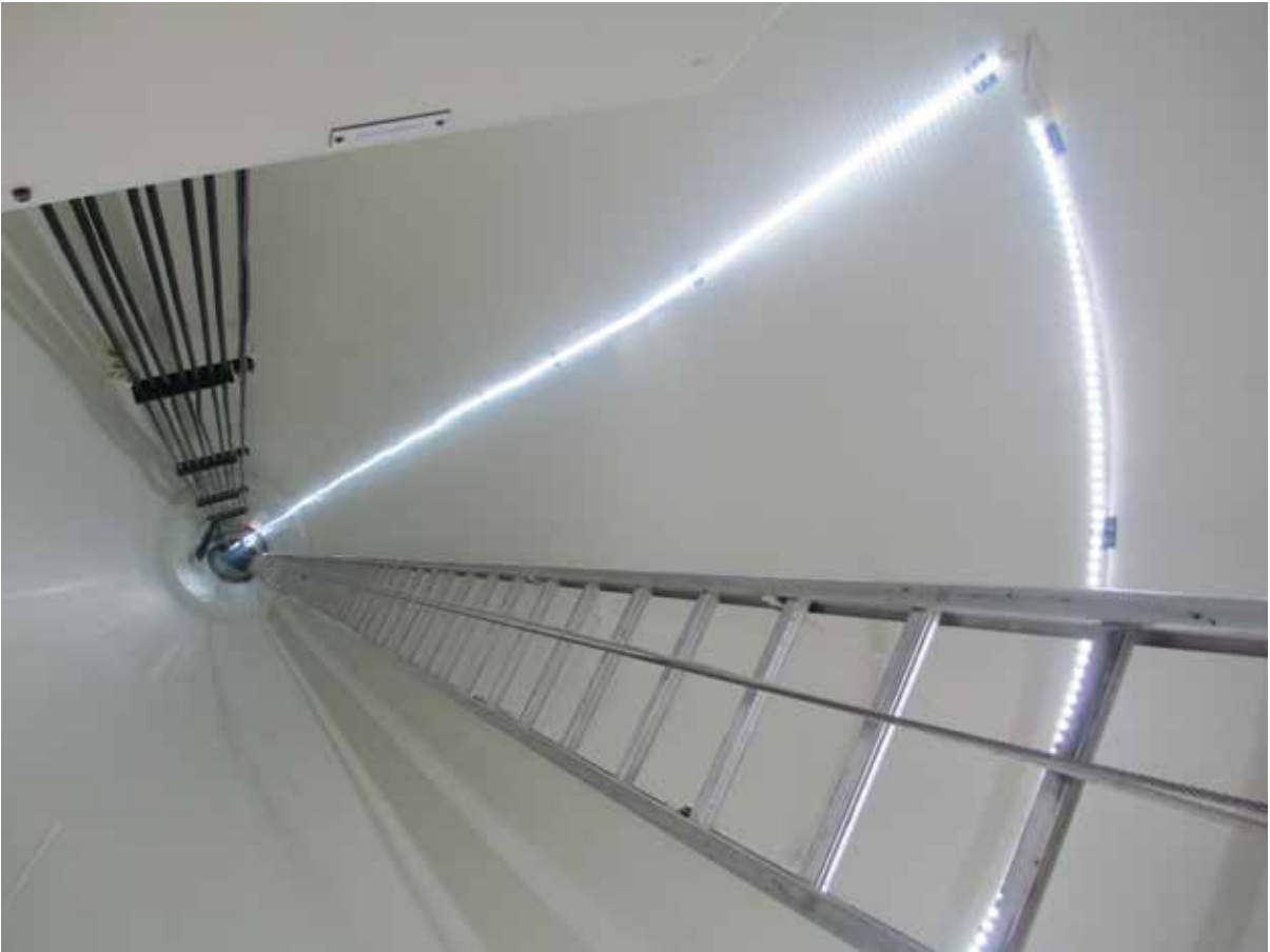
LongRun Strip Light inside wind turbine shaft
